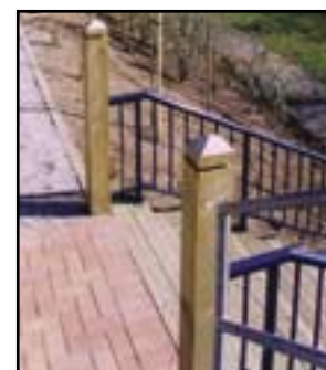
Stair System – Heritage Woods, Port Moody, B.C. photo credit: Donna Rodman
